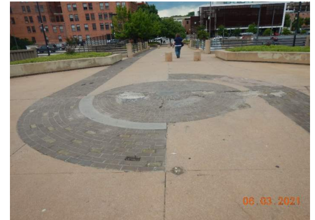
Example of pavement to be patched / repaired
