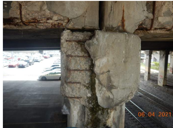
Example of below-deck concrete to be repaired
